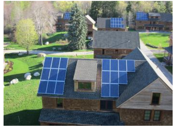
Photovoltaic solar panels purchased in a community volume purchase. KW Management of Nashua, NH installed the systems at Nubanusit Neighborhood & Farm Cohousing, Peterborough, NH 2010-11. www.peterboroughcohousing.org
