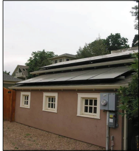
Solar panels placed on an accessory structure not visible from the public right of way should still follow the slope of the roof and have a low profile. Photo courtesy of Dan Corson
