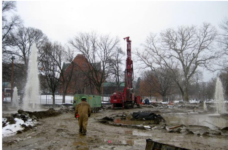
Figure 5 – The importance of knowing the layout, history and underlying geology of the project site, The above photo shows multiple geysers created when air rotary drilling encountered paleokarst. The air forced ground water up previously drilled boreholes, and the project site quickly became mired in mud. In southwestern Ohio a business owner preparing to install an open-loop system on a commercial property discovered the property was a former gas station with ground water contamination. Discharging the contaminated water into the Great Miami River, as originally planned, would have subjected the owner to costly legal fees and cleanup costs.
