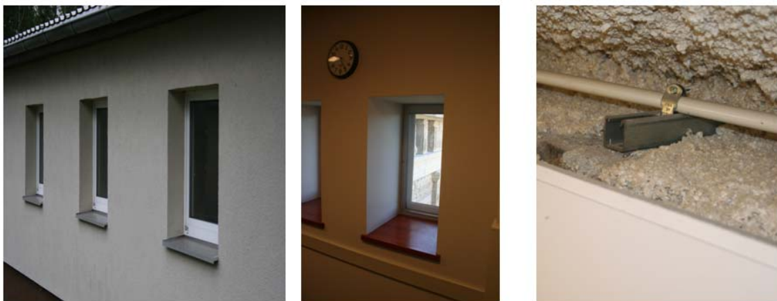
Figure 2. Retrofitted Army barracks with exterior insulation (left), interior insulation of the retrofitted administrative building at the Rock Island Arsenal (center, right).
